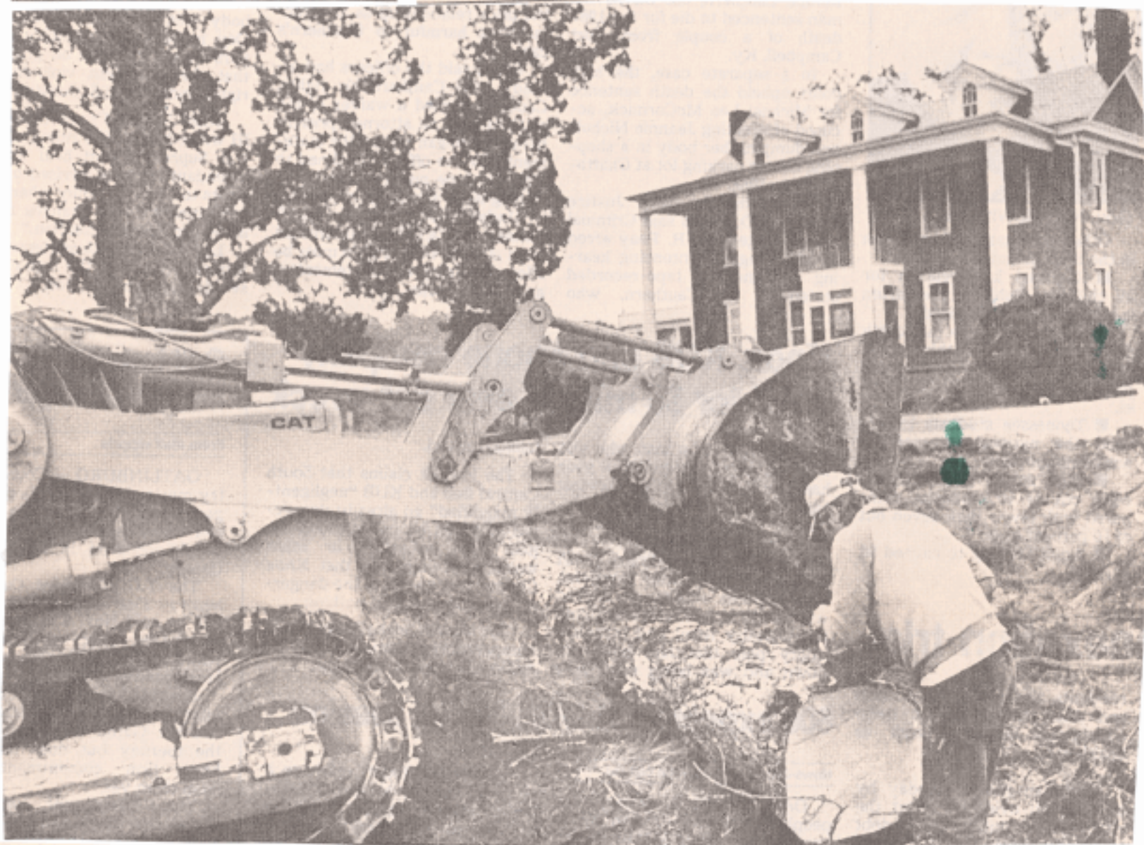
Workers cut down trees on the front lawn of the Baker-Peters House as part of a compromise plan to save the house and still allow Phillips Petroleum Co. to develop a gas station and car wash on adjoining property. Already felled was an 85-foot-tall rock elm, the state champion — tied with another leafy giant as the largest of its species in Tennessee.
